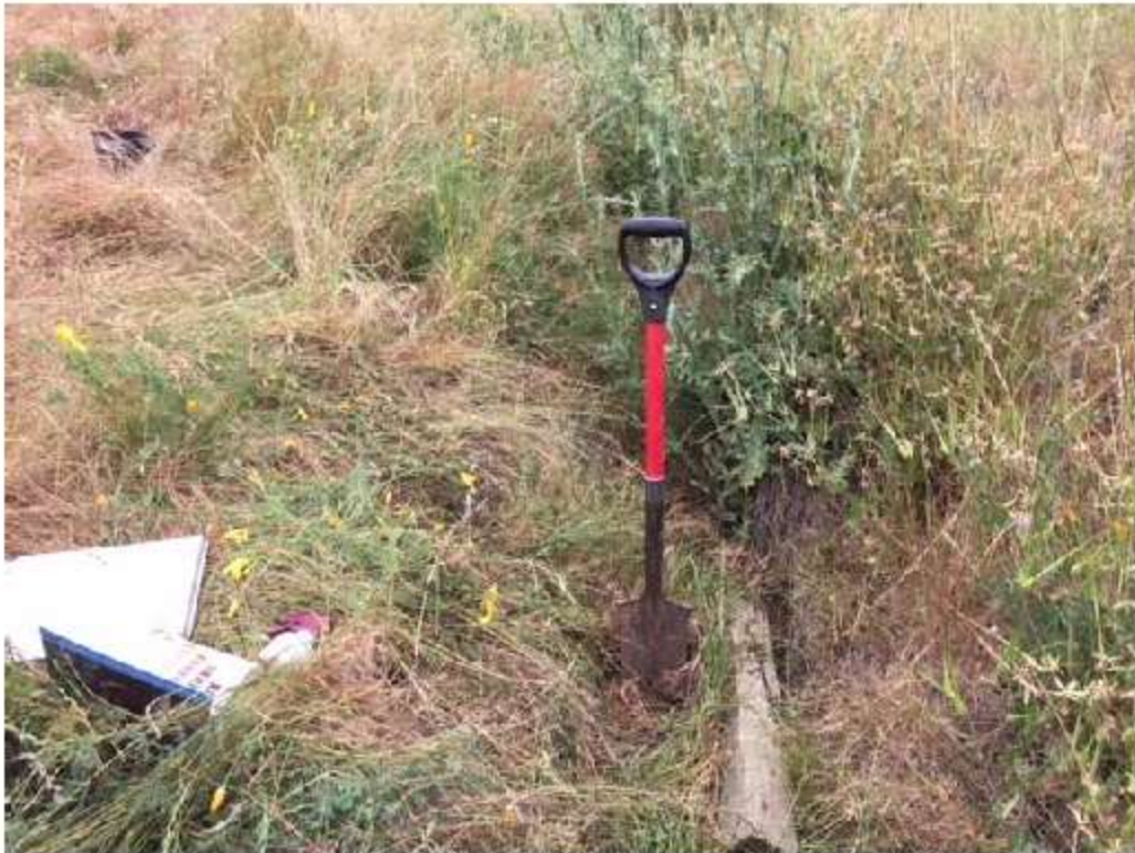
Appendix C-4. Man-made drainage ditch lacking an OHWM and positive indicators of all three wetland parameters at Sample Point 3.
